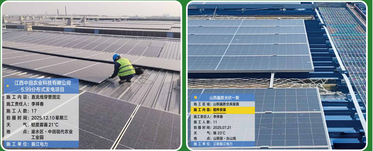
The 5.99MW rooftop distributed photovoltaic project of Jiangxi Zhongtian Modern Agricultural Technology Co., Ltd. and the 2.56MW rooftop distributed photovoltaic project (Phase I) of Yingsheng Ceramic Fiber in Shuozhou, Shanxi Province
